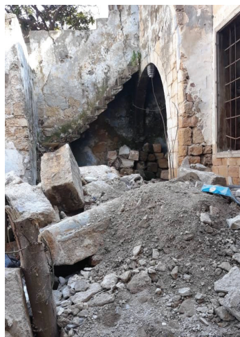
A damaged neighbourhood in Jableh
